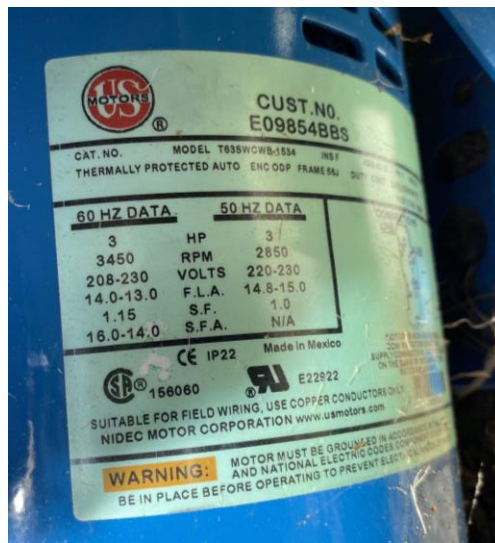
Figure 4: Nameplate of a Three HP Pump with no VFD.
