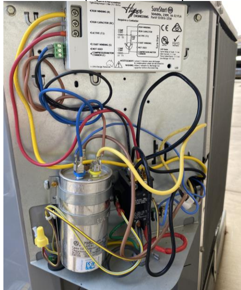
Figure12: Air conditioner wiring compartment with soft starter installed
