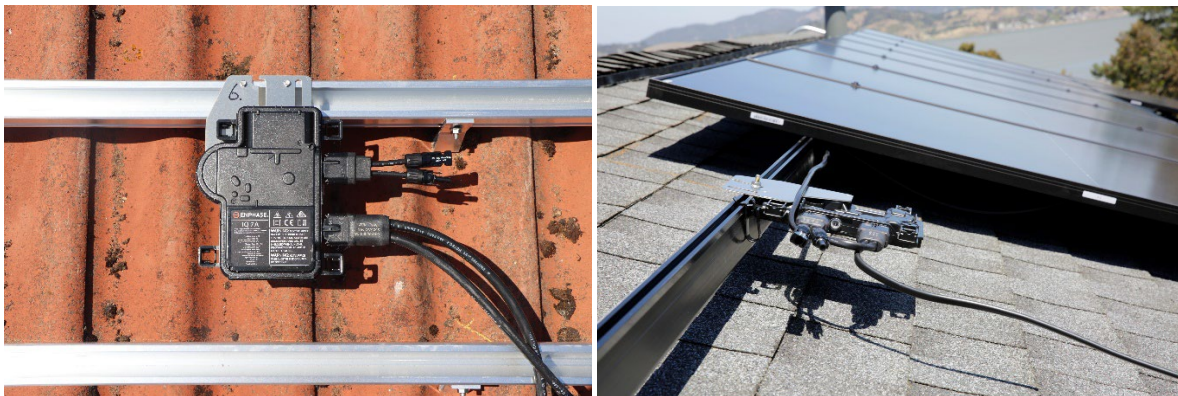
Figure 1: Enphase microinverter system
