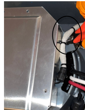
Figure 1: Zigbee Antenna tied to the side of the E3 cover
