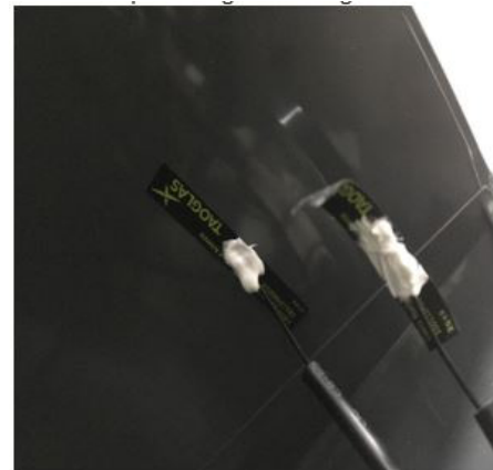
Figure 7: Removing damaged Zigbee antenna
