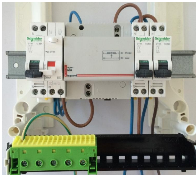
Figure 9: Legrand Filter Fitted in a Single Phase Distribution Board/Load Centre
