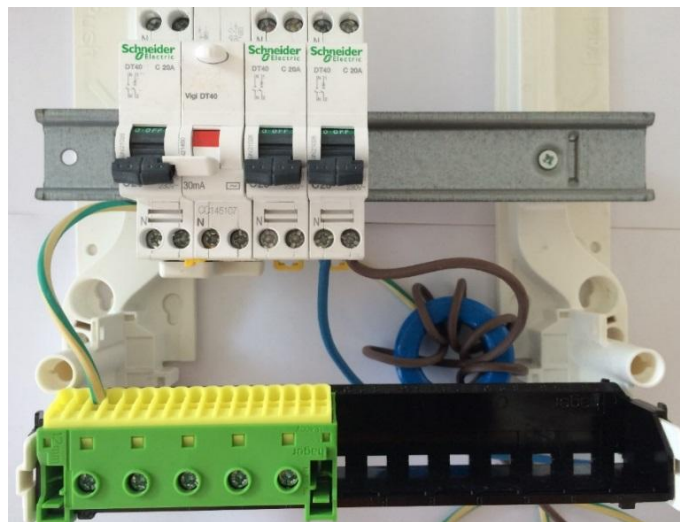
Figure 8: Toroid Rings Fitted in a Single Phase Distribution Board/Load Centre
