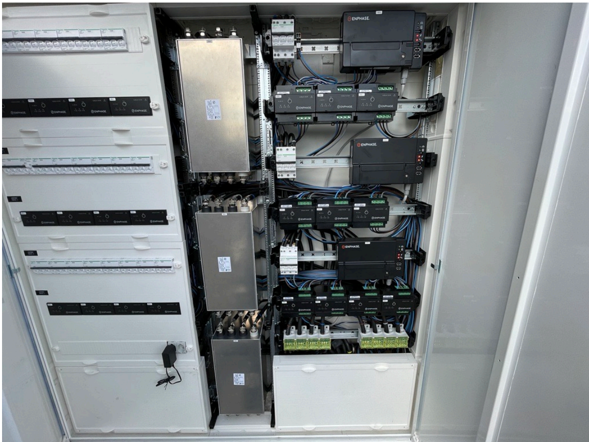
Figure 12: Example of a PLC filter usage in a commercial environment with three Radius LCF-250-PC 250 A filters to separate the communication domains for three IQ Gateways
